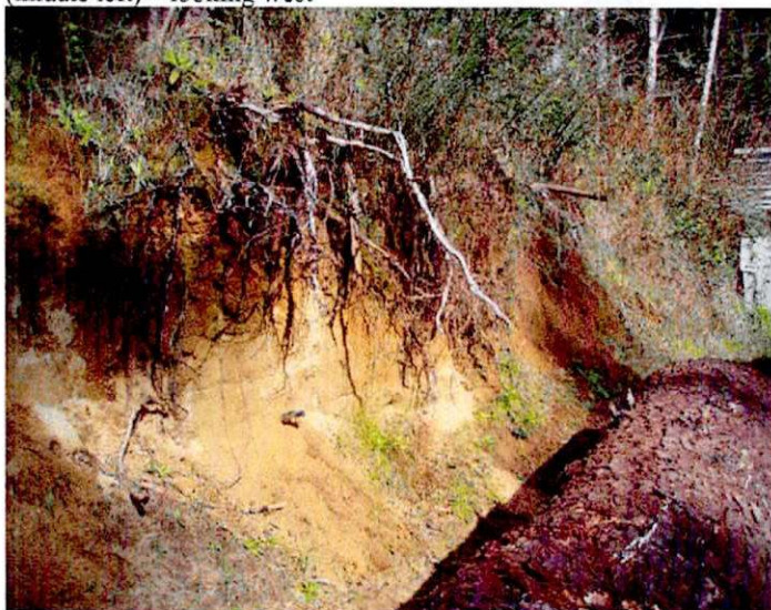
Close-up of cut bank.
