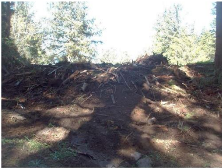
Soil and slash fill at south end of cleared portion of the site – looking north.
