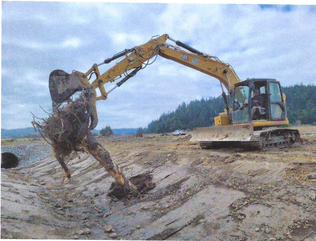
Figure 4. Installation process of LWD at an SWCD/ODFW project tidal channel, North Bank Working Landscapes Project, in September 2023. Stem is pushed fully into the soil until rootwad is at ground level. The stem with soil friction provides maintains LWD stable in place.
