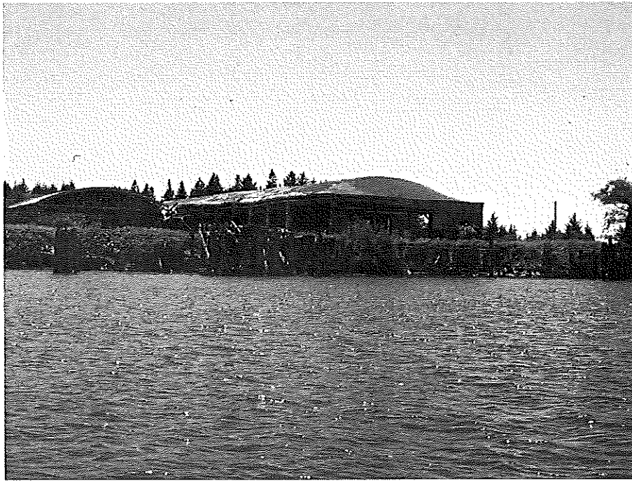
Figure 22. Rogge Mill shortly before demolition, 2019. Photography courtesy of Jim Proehl, Bandon Historical Museum.
