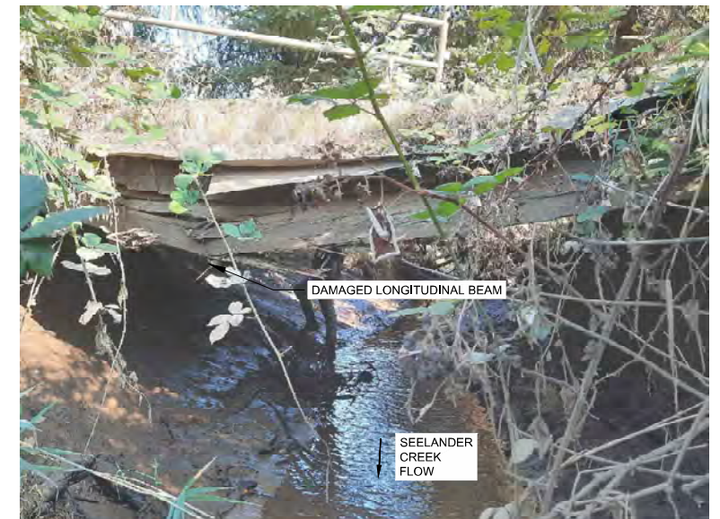
5 EXISTING BRIDGE - LOOKING UPSTREAM AT DAMAGED LONGITUDINAL BEAM Scale: NTS
