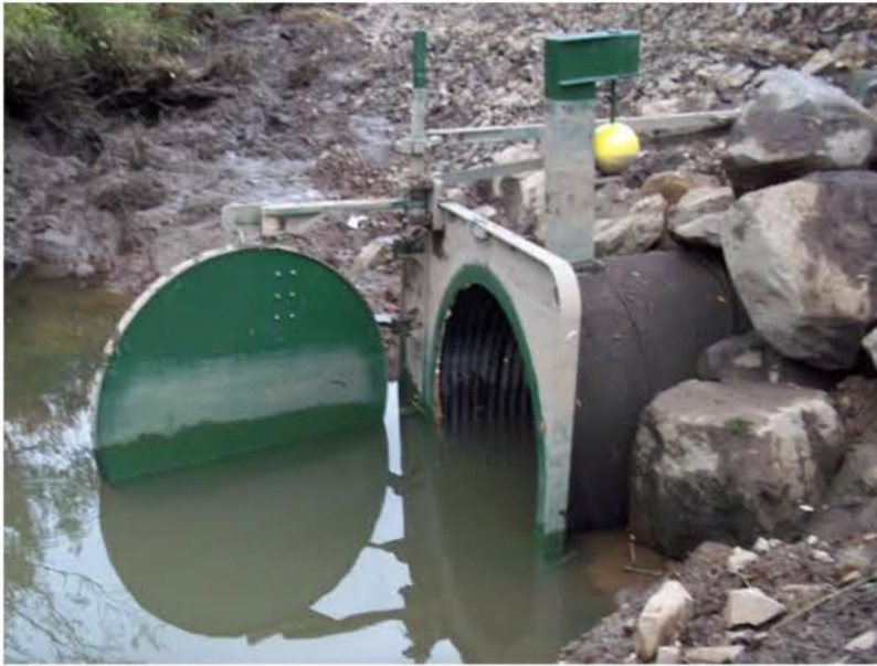
Figure 4. Side-hinged aluminum tidegate door in working location.
