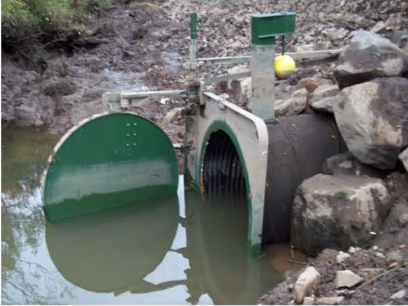
Figure 3. Side-hinged aluminum tidegate door in working location.
