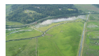
TIDAL GATE CURRENTLY IN DISREPAIR IN THE COALEDO DRAINAGE DISTRICT. (PHOTO CREDIT: LUKE FITZPATRICK)
