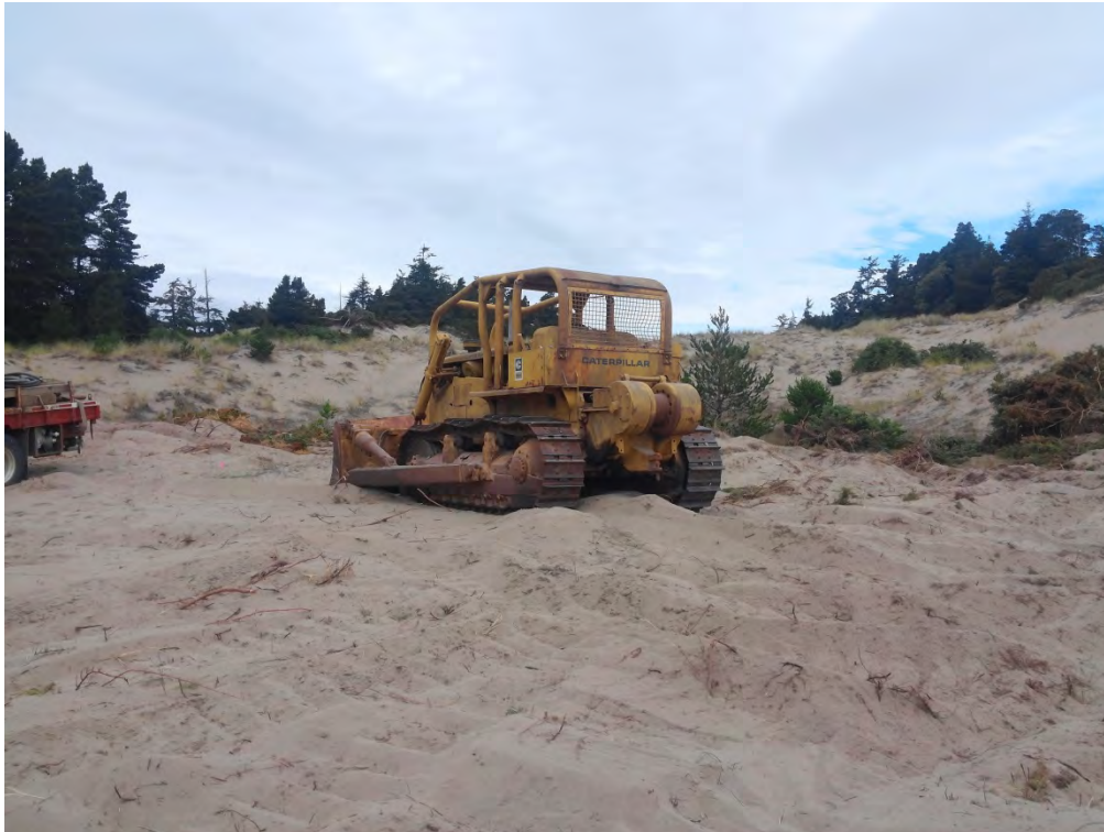
Bulldozer used to plow and cut trails and push down trees and shrubs.
