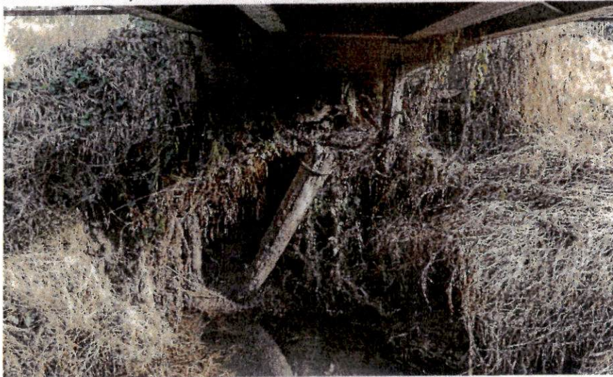
Figure 4: Steep unprotected bank below Bent 1 abutment
