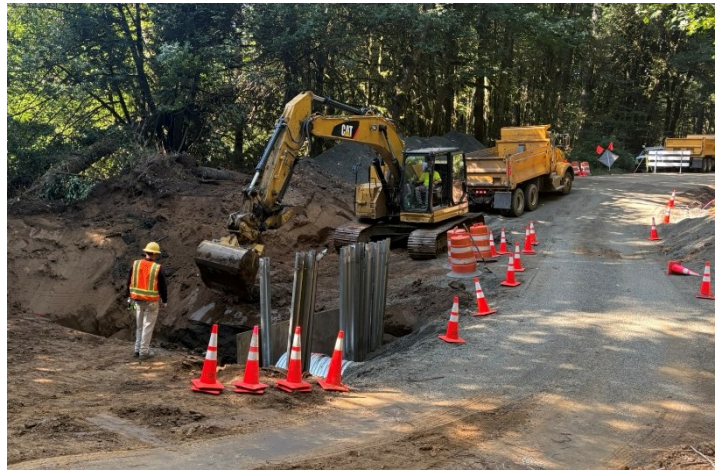
Culvert replacement on the Coquille-Fairview Road conducted by Coos County Roads Department in September 2025 will support movement of threatened and endangered fish. Culvert replacement and maintenance can also create more fire-adapted roads that can handle post-fire sedimentation.
