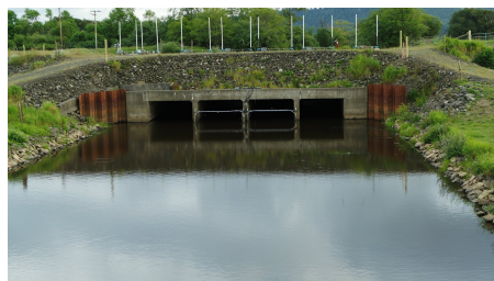
TIDE GATE FOR BEAVER SLOUGH DRAINAGE DISTRICT. (PHOTO CREDIT: LUKE FITZPATRICK)
