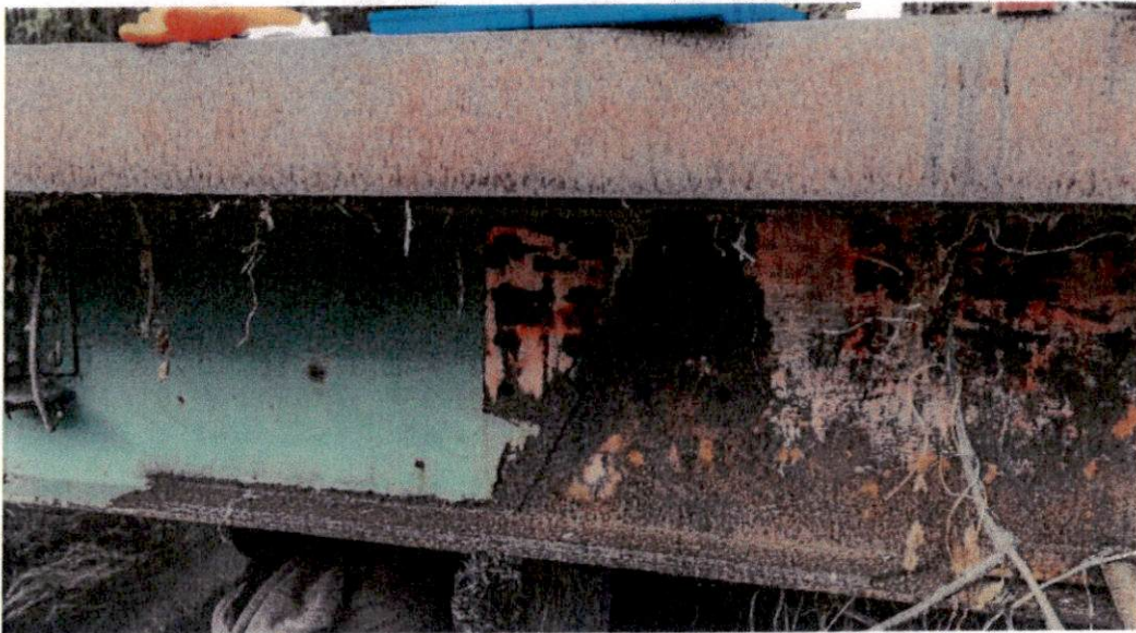
Figure 3: Exterior girder (Type 1) with areas of paint failure
