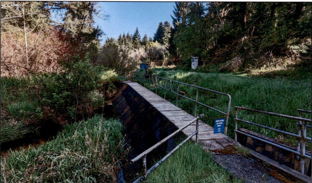
Figure 8. Existing conditions of the downstream bar grate and crossing (Station 211.5 ft). The bar grate is skewed approximately 60 degrees to the channel.
