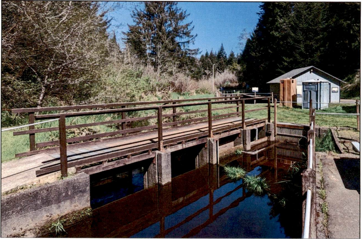
Figure 7. Existing conditions of the weir and footbridge (Station 423.5 ft). The proposed project is immediately upstream from the weir on the floodplain north of Ferry Creek.
